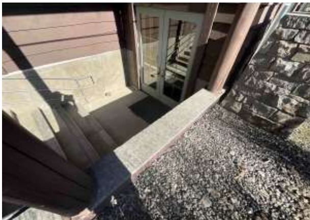
Missing guardrail; code non-compliance
