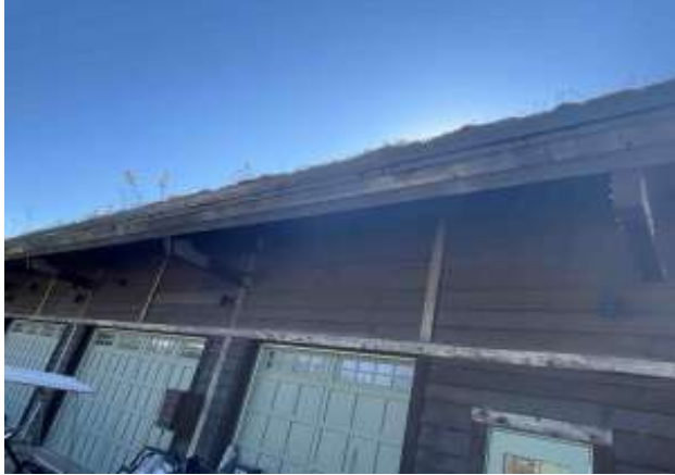
Moss growth at roof edges
