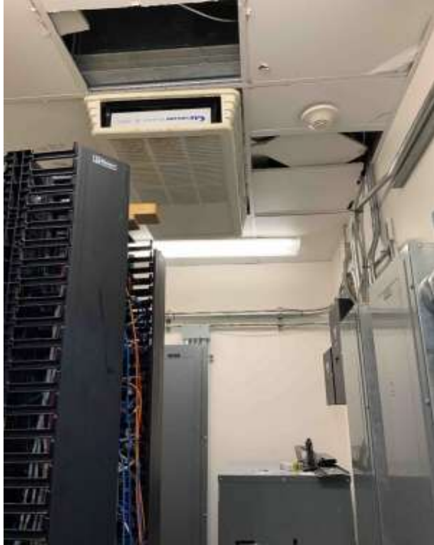
Example of missing /damaged ceiling tiles
