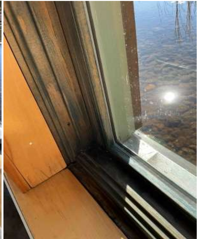
Evidence of water infiltration at sills
