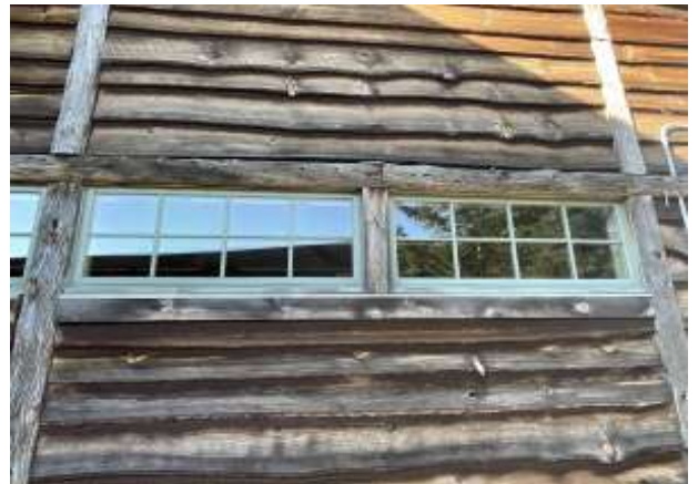
Damaged window sill trim
