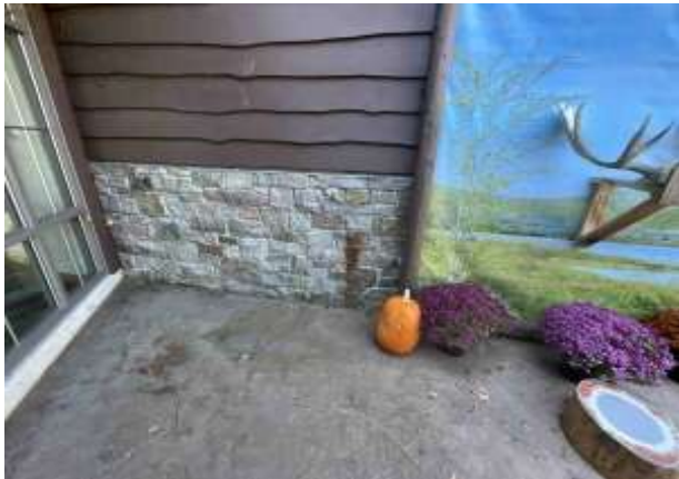
Example of stained stone façade
