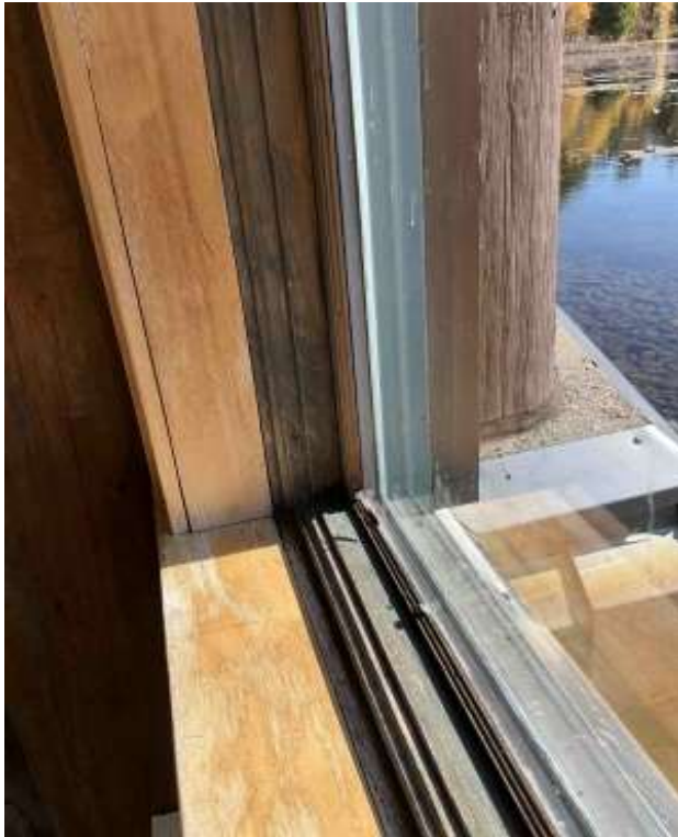
Example of worn window finish
