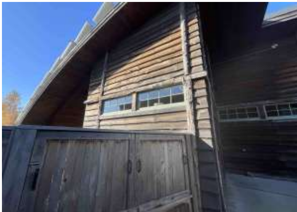
Damaged timber trim
