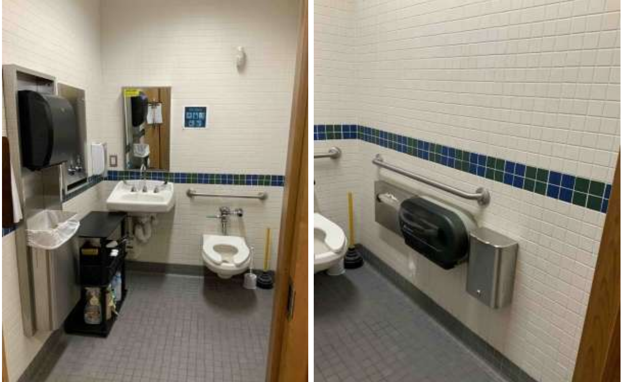
Unisex toilet in admin area
