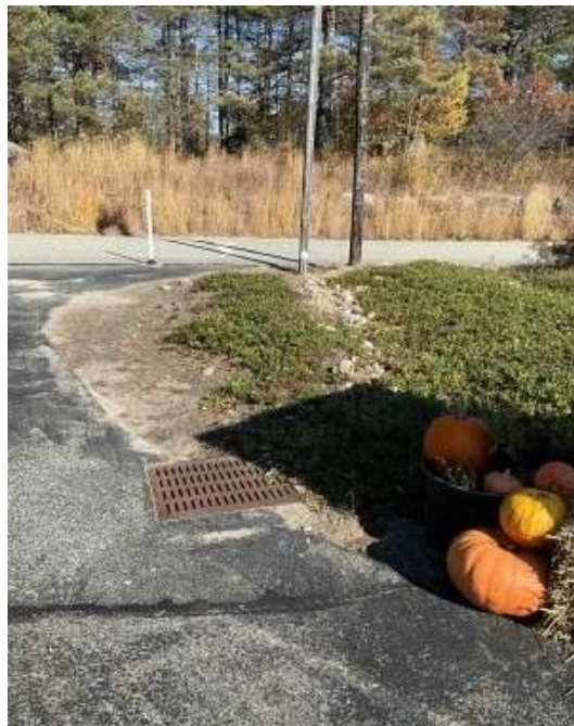
Figure 2 Stormwater drainage near ADA drop off
