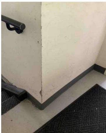
Example of area requiring patch/paint
