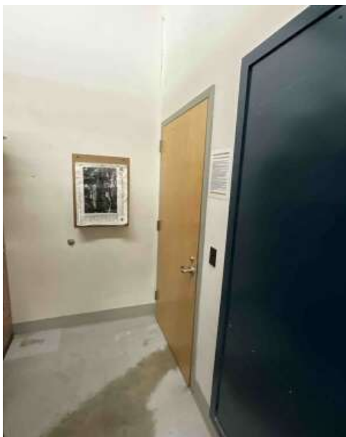
Garage interior fire door
