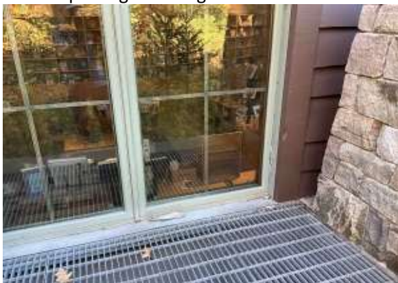
Example damaged window weatherstripping at exterior
