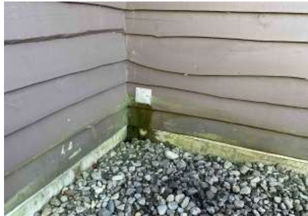
Example of assumed moisture damage
