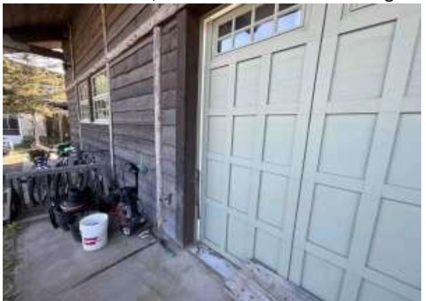
Damaged jamb trim at 108B
