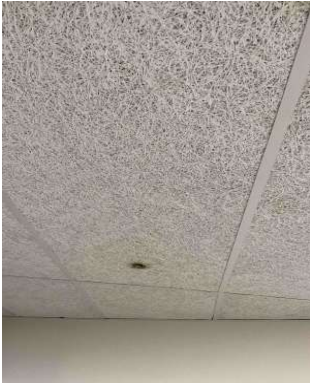
Example of damaged ceiling tile
